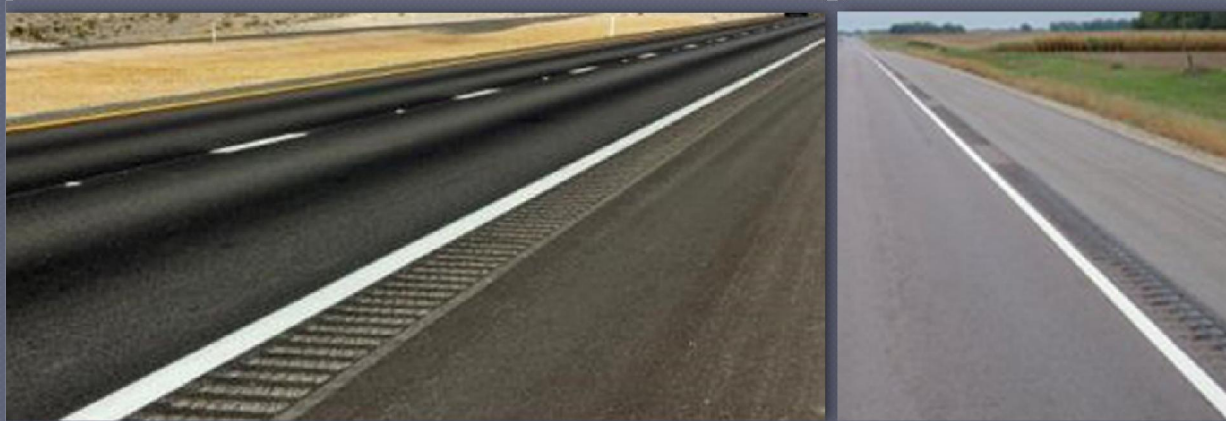
Shoulder Rumble Strips
